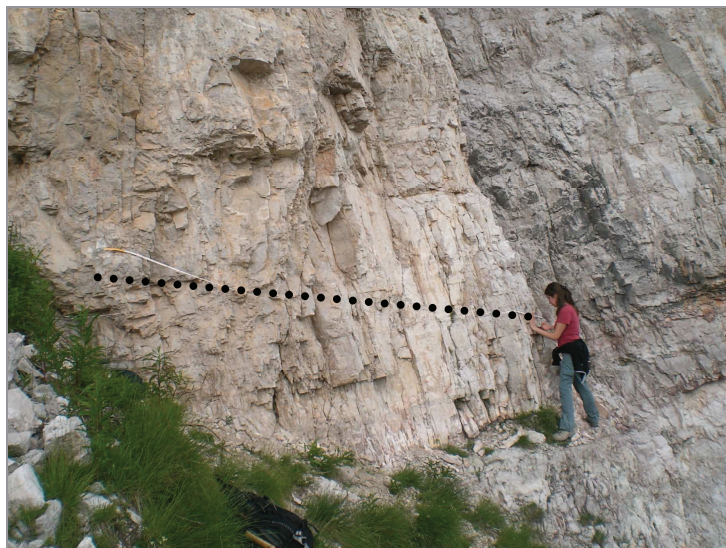
Fig. D.2. Approximate position of the horizontal scanline at the basement of the western side of the Torre Grande: Site 1. The trace of the scanline is drawn-in by hand. The horizontal scanline survey was done from left to right over 5.00 metres.
