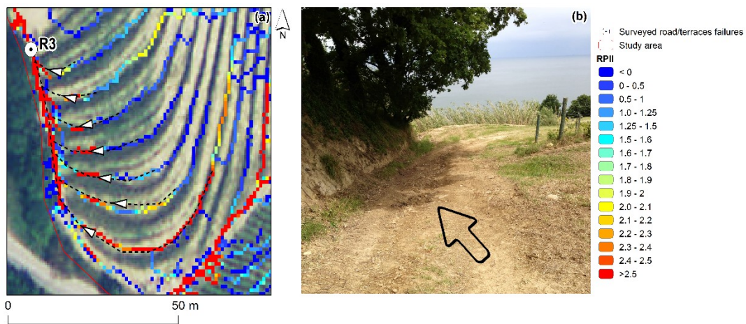
Figure 7. Pesaro case study. RPII maps derived from the 1-m ALS DTM (a) highlighting the flow modifications induced by the terraces, causing water accumulation that erodes the road (b).
