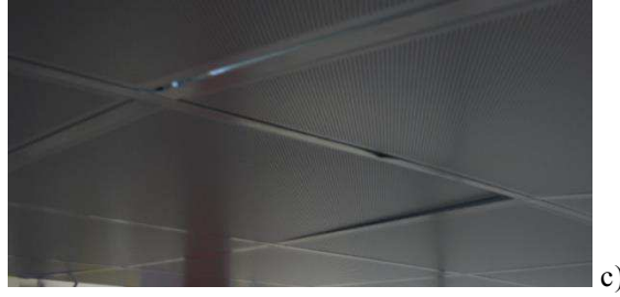
Fig. 51: Damage mechanism of T-Grid with Metal tiles after cyclic test: a) buckling phenomena on the slotted studs of seismic bracings, b) lift of the main runner and rotation of the bracket of the seismic bracing, c) uplift and slight dislodgement of tiles in the area close to the seismic bracing.
