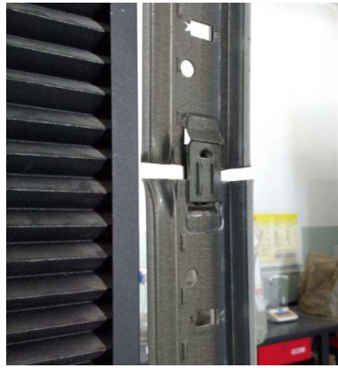
Fig. 26: Detail of damage of the dimple.
