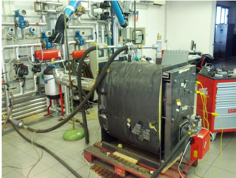
Figure 1.2.1.1. Picture of the heat generator used for the experimental analysis.
