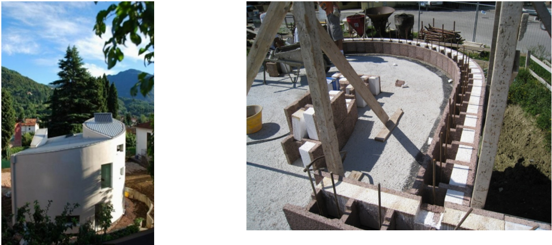
Figure 2-2. Residential building with curved wall surface (left), the first line of blocks (right)
