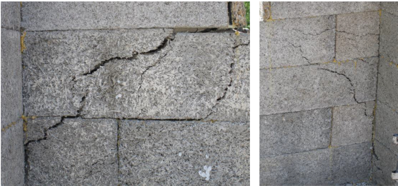
Figure 10-5. Diagonal cracks on the upright ends in a wall with window
