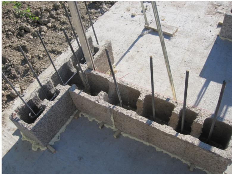
Figure 2-4. First line of blocks with the starting bars anchored in the foundation
