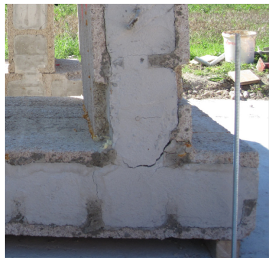
Figure 11-10. Specimen 11 at failure
