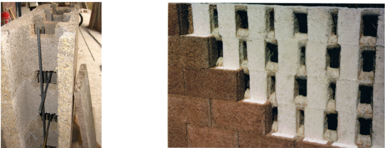
Figure 2-3. Reinforcement inside the wall before casting (left) and internal RC grid (right)
