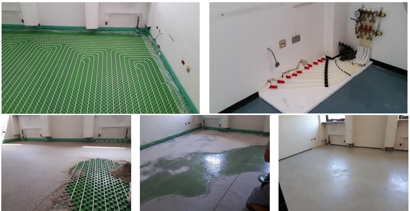
Figure 6.10 - Installation of the floor radiant system and making of the resin flooring.
