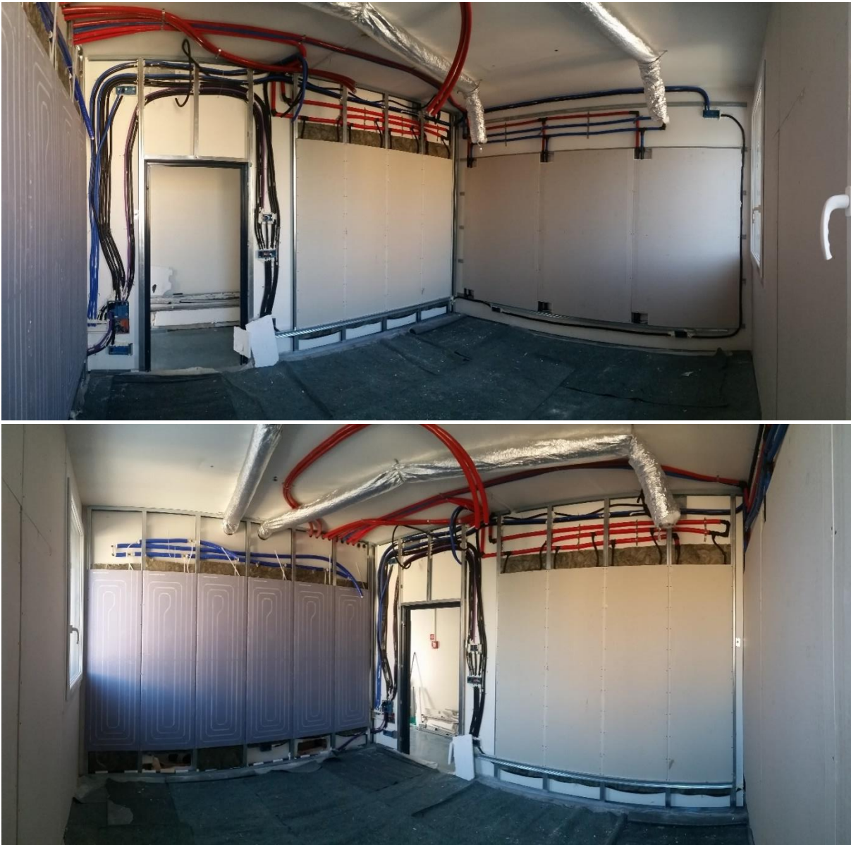
Figure 6.15 - Views of the room with the hydraulic connections of two walls completed.
