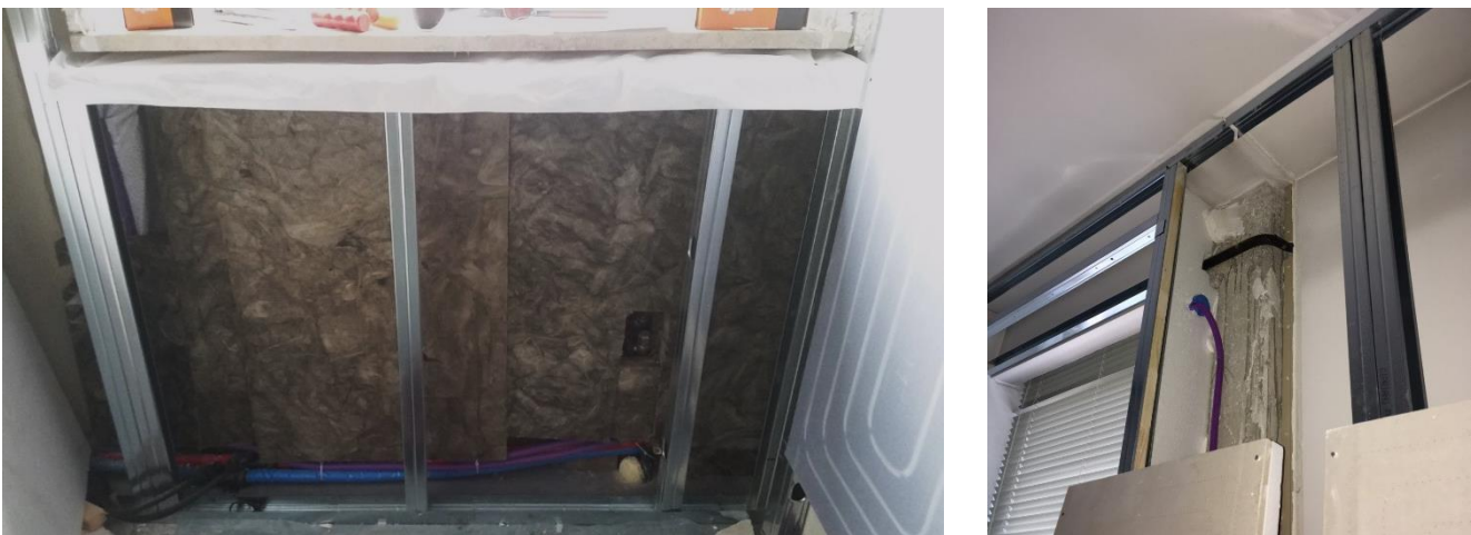
Figure 6.12 - Details of the external wall: position of the hydronic connections, insulation of the recess under the windows and electrical set-up for the new Venetian blinds which will replace the old ones which are still present.
