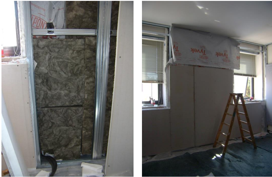
Figure 6.13 - Details of the external wall: insulation of the space behind the dry wall, with a vapor barrier placed on the existing external concrete wall and a vapor barrier immediately behind the radiant panels.
