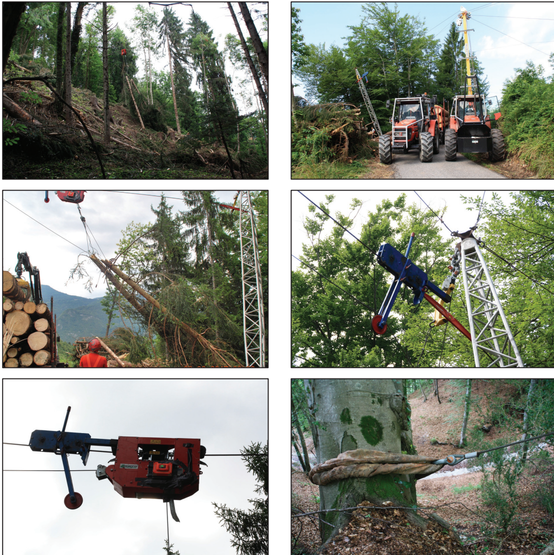
Figure 6.6: Photos of Site F. From the top left: Inhaul; Landing; Unloading; Artificial support; Carriage; Anchor
