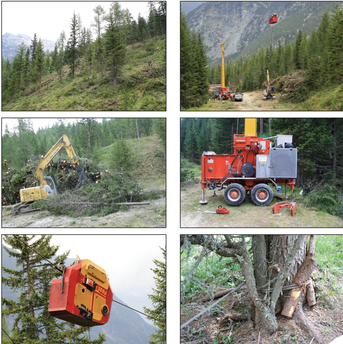
Figure 6.11: Photos of Site M. From the top left: Harvested area; Landing; Unloading; Cable yarder; Carriage; First of the in-line double anchor
