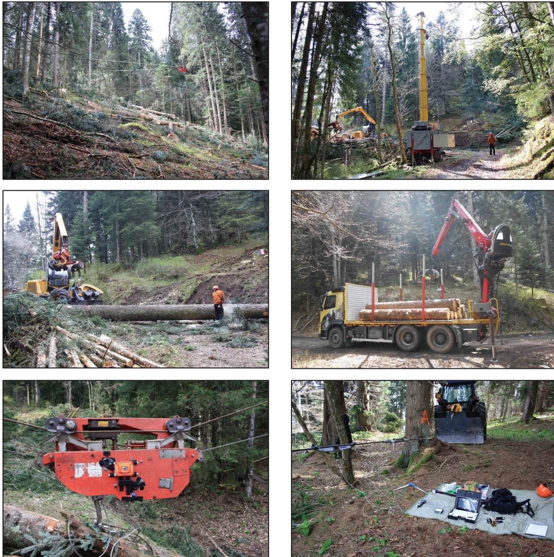
Figure 6.1: Photos of Site A. From the top left: Loading area; landing, Log processing; Log truck; Carriage; Anchor
