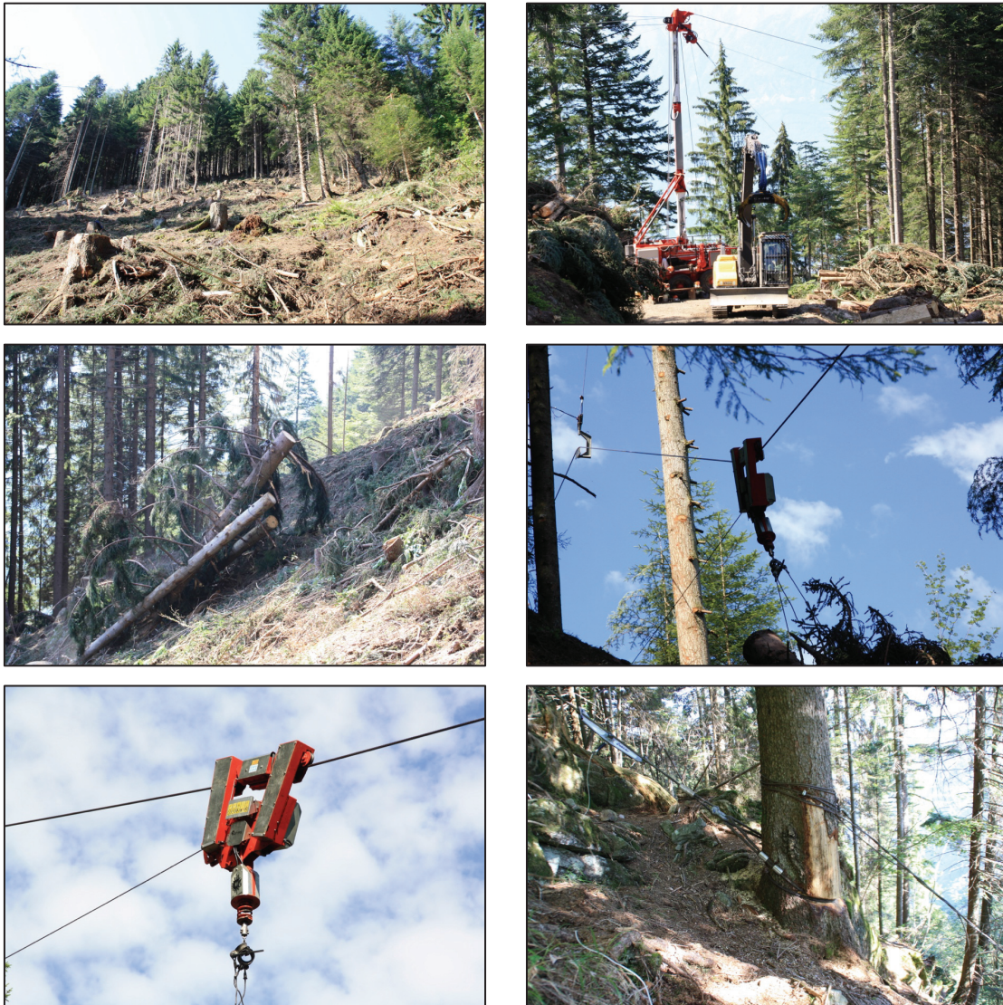
Figure 6.9: Photos of Site I. From the top left: Loading area; Landing; Lateral skid; Inhaul; Carriage; Anchor
