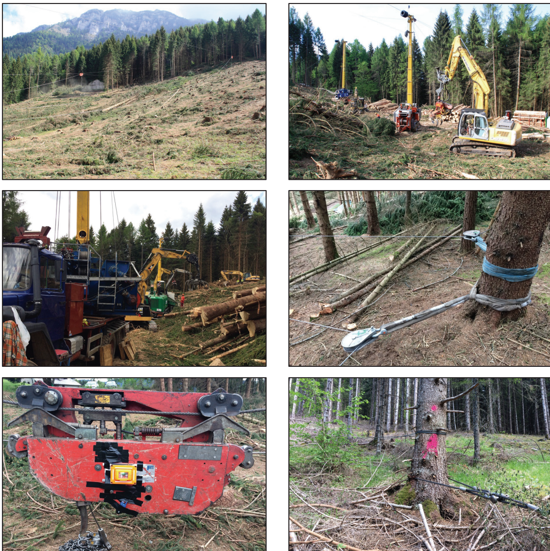
Figure 6.3: Photos of Site C. From the top left: Loading area; Landing; Machine operating at the landing; Haul-back line shared supports; Carriage; Anchor
