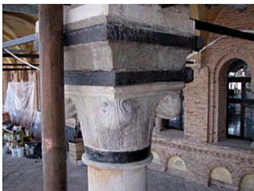
Figure 2.38: Integration of the original metallic confinement on a capital in Palazzo della Ragione, Padova (Valluzzi 2008)
