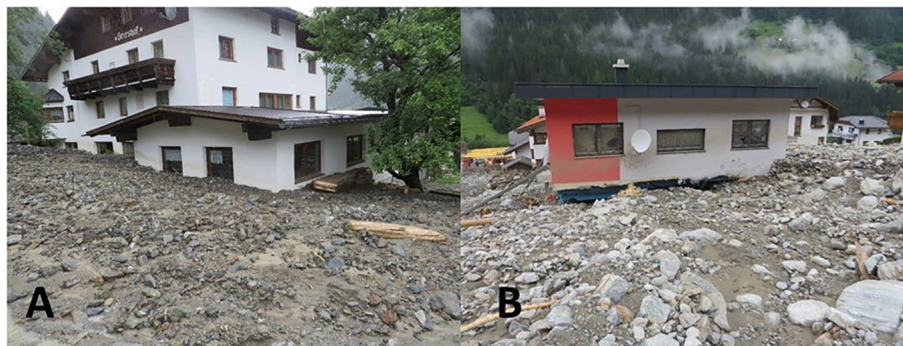
Fig. 9. Two buildings that experienced the highest degree of loss (approximately 1) in the Schallerbach case study (Source: WLV).
