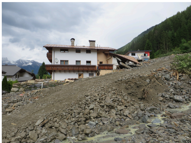
Fig. 2. Damaged buildings in Schallerbach (Tyrol, Austria). The building is located on the slope and, for this reason the deposit height is very high at the back side of the building in comparison with the deposit height observed in the opposite side. (Source: Austrian Service for Torrent and Avalanche Control, with permission).
