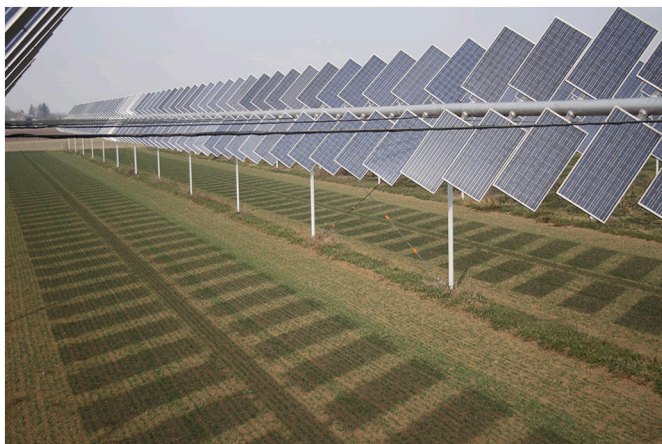
Fig. 3. APV plant in Borgo Virgilo (Lombardia region) © 2020 REM TEC s.r.l.
