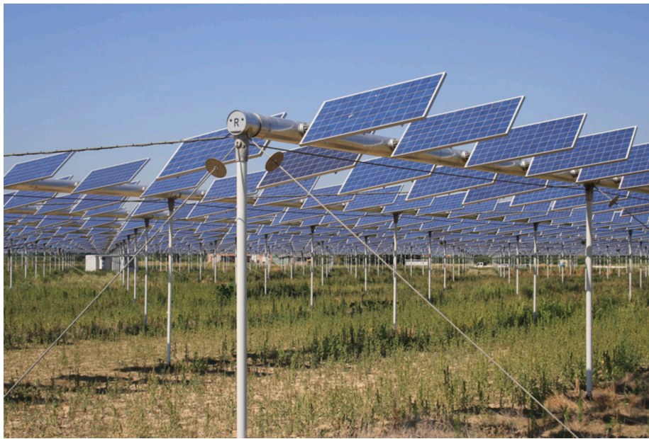
Fig. 1. APV plant in Castelvetro (Emilia-Romagna region) © 2020 REM TEC s.r.l.
