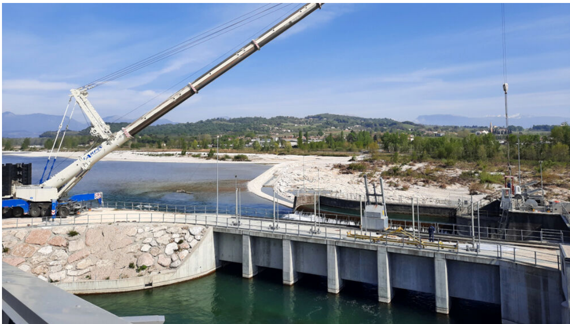
Figure 11: Nervesa della Battaglia hydraulic intake work.
