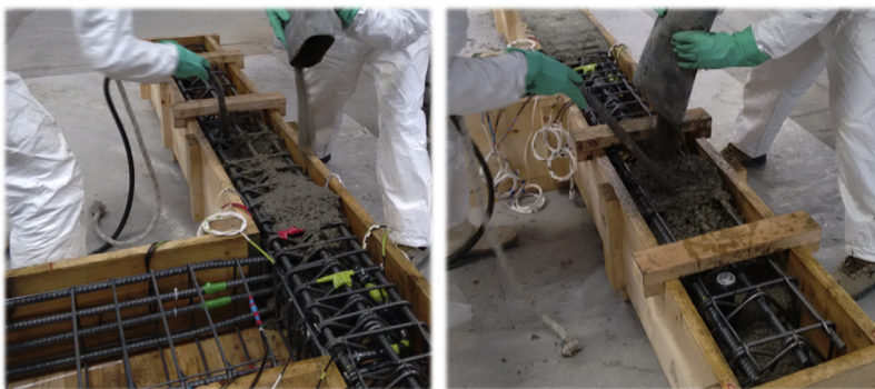
f0020 Figure 2.3 Casting operations of concrete with electric arc furnaces (EAF) slag aggregate.
