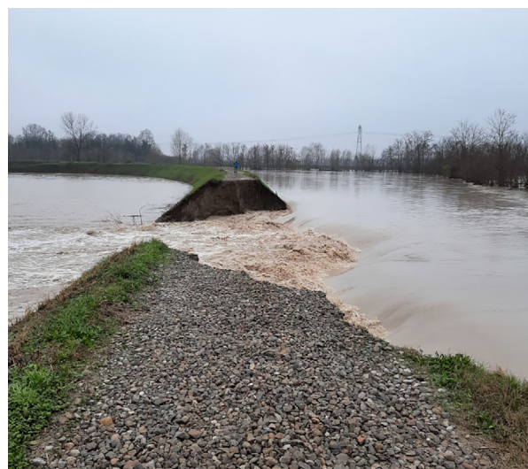
FIGURE 2 Photo of the breach at 8:40 on 6 December.
