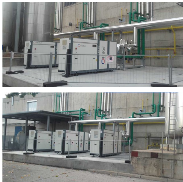
Figure 3.4 Heat pumps of the CCC supply station. (Courtesy of AGSM).
