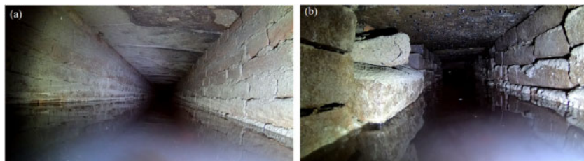
Figure 4. Inner view of two drainage conducts in S. Mark's square: (a) gatolo in good conditions, (b) gatolo in bad conditions.
