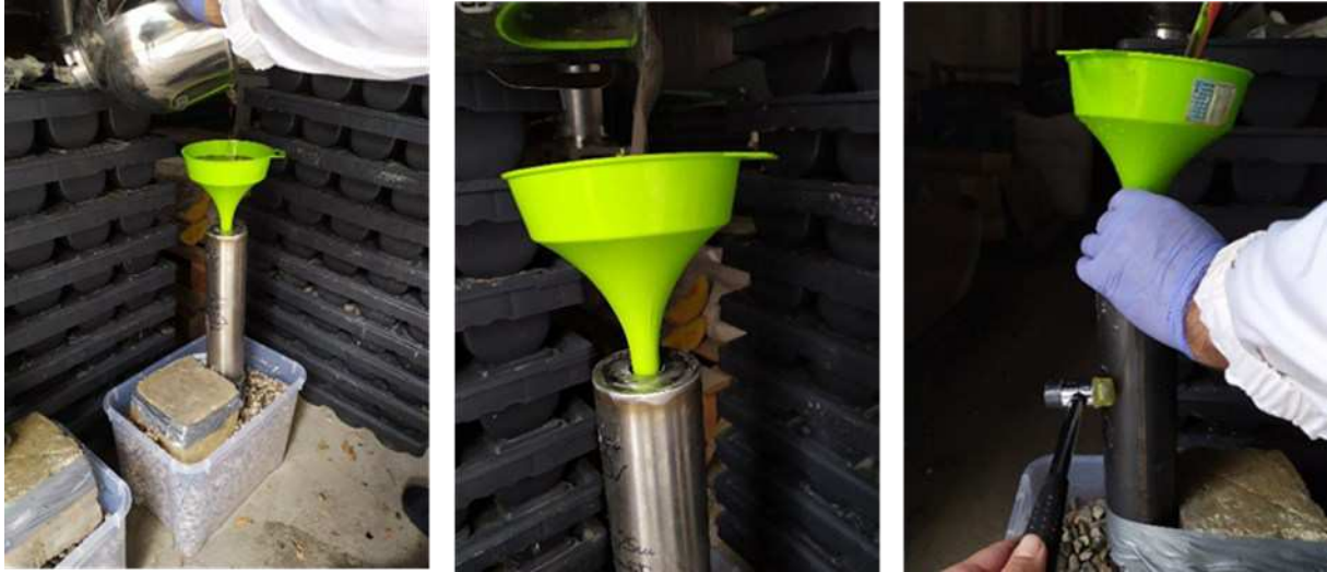
Figure 23: From left to right, SV inserted into the well point, a detail of the low viscosity of the material, use of the hammer to enhance the grout descend.
