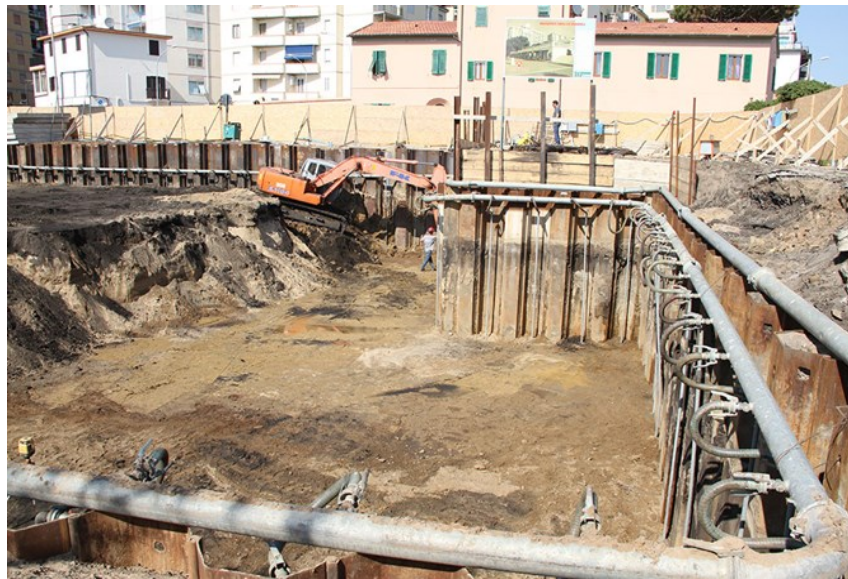
Figure 5: Example of well point dewatering system around an excavation for building foundation.
