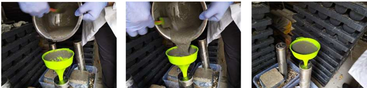
Figure 26: From left to right, MF928 inserted into the well point, a detail of the higher viscosity of the material, detail of the filling operation.
