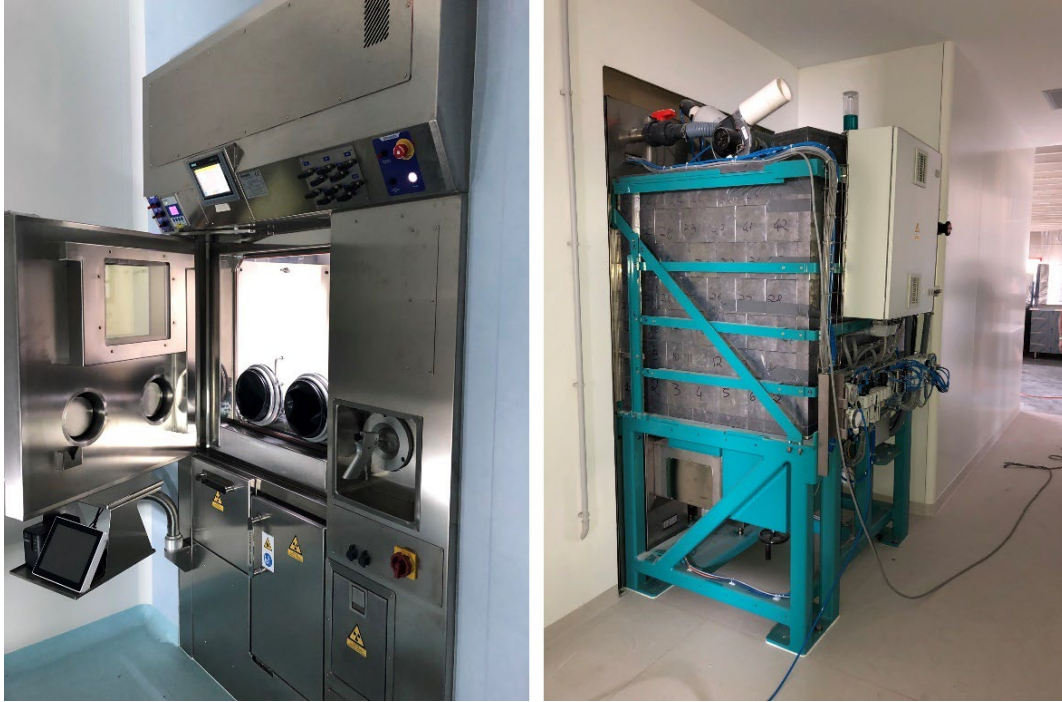
Figure 15. Hot-cell installed in the LARAMED facility. The lead shield is visible on the back side of the hot-cell (right).
