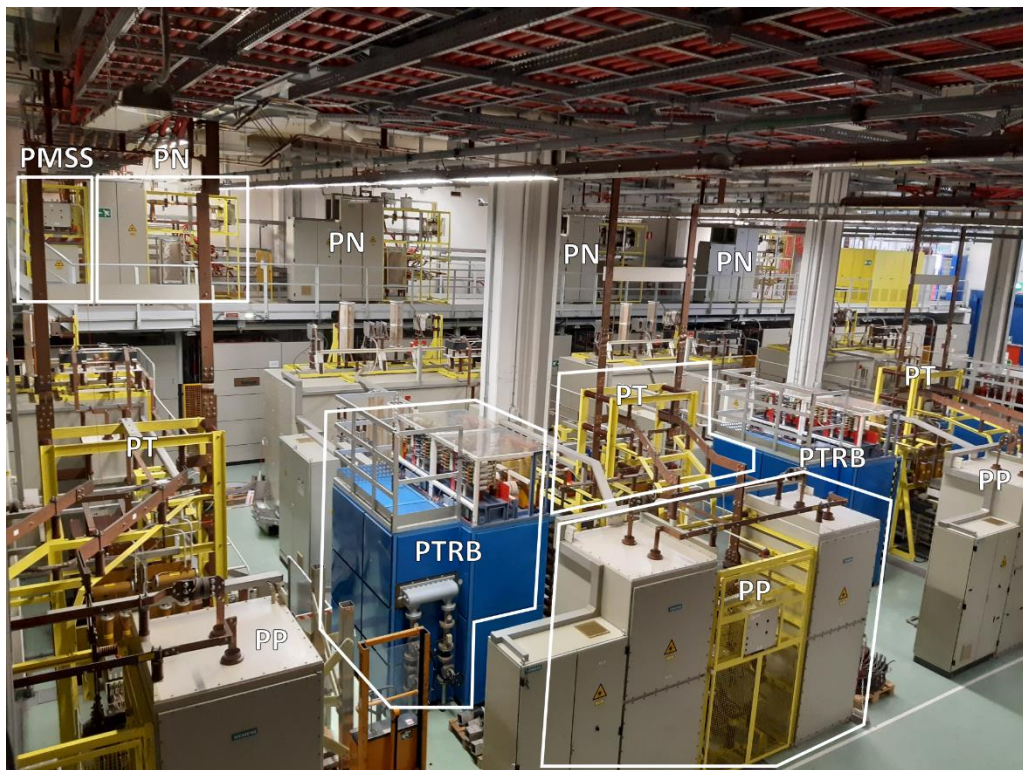
Figure 20 – RFX-mod power supply hall
