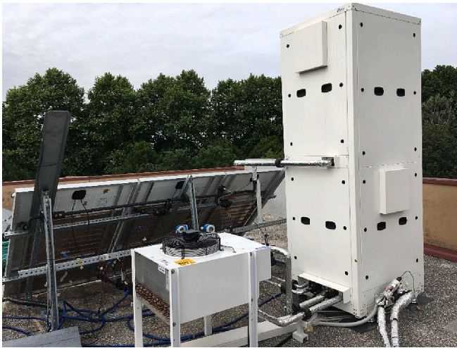
Fig. 2. Picture of the heat pump prototype, including finned coil evaporator and PVT collectors.
