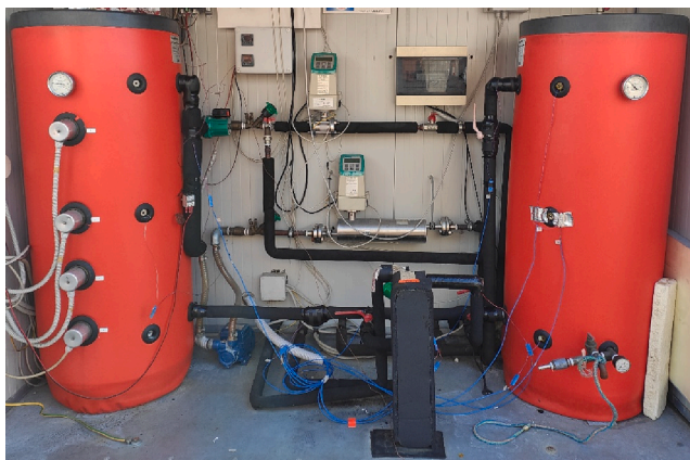
Fig. 3. Picture of the water tanks and the USER brazed plate heat exchanger.
