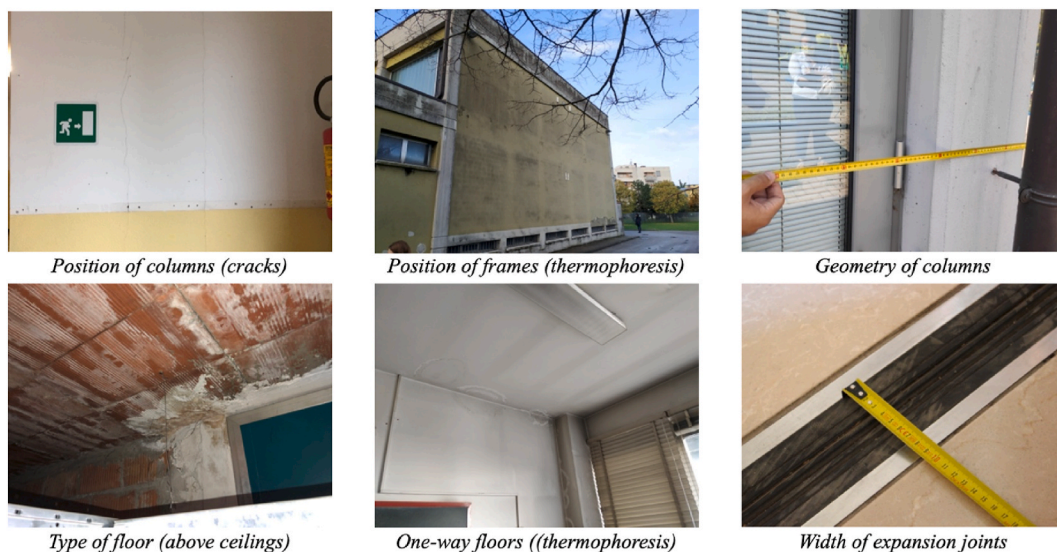
Fig. 1. Information gathered through visual inspections.
