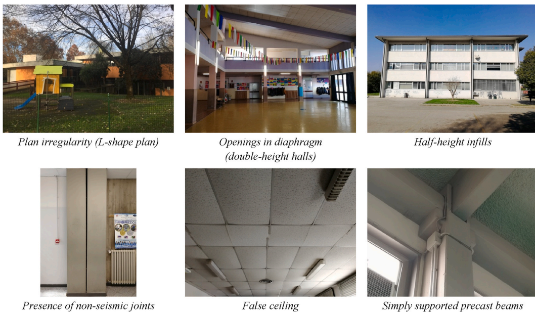
Fig. 15. Commonly observed deficiencies in the analysed stock.
