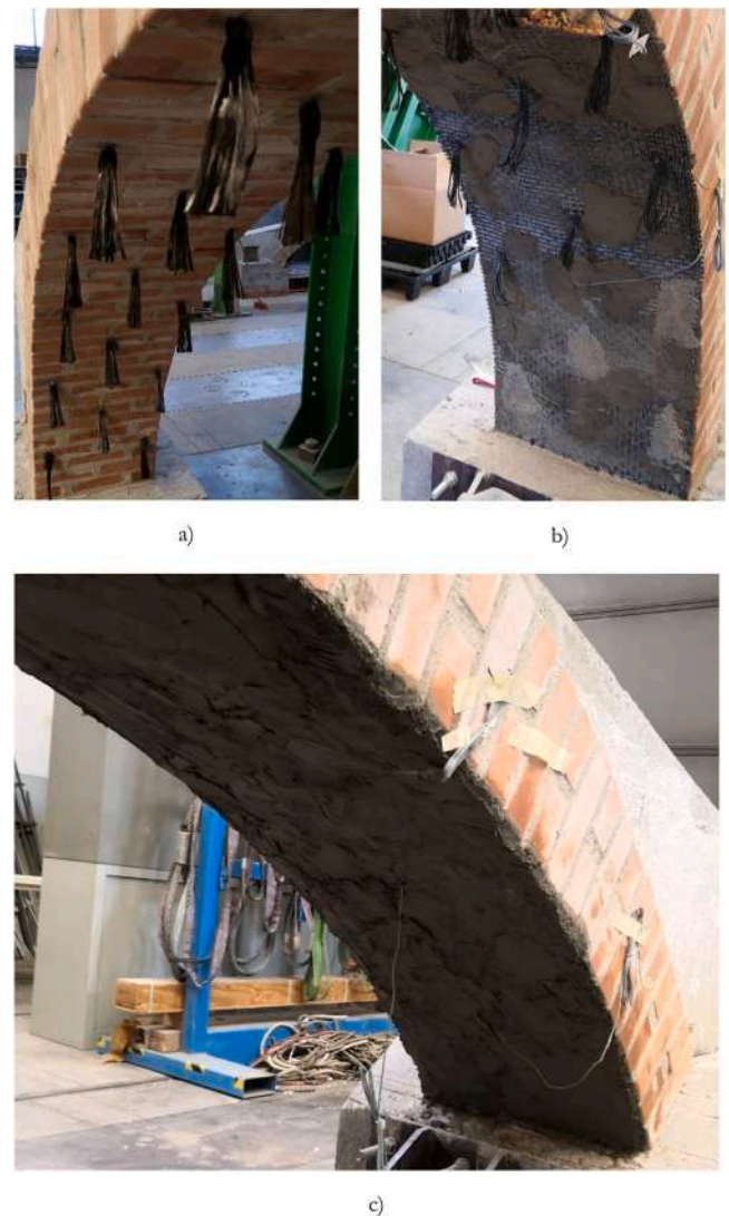
Fig. 3. Application of the strengthening system: a) Application of the spike anchors; b) application of the first layer of mortar and the fiber strip; c) application of the second layer of the matrix.
