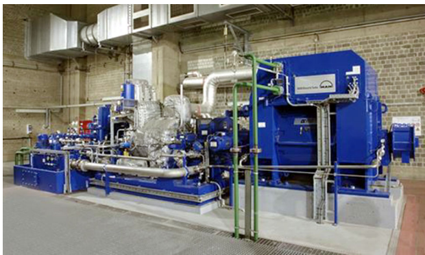
Fig. 4 Example of a small size steam turbine (courtesy of Man Diesel and Turbo)
