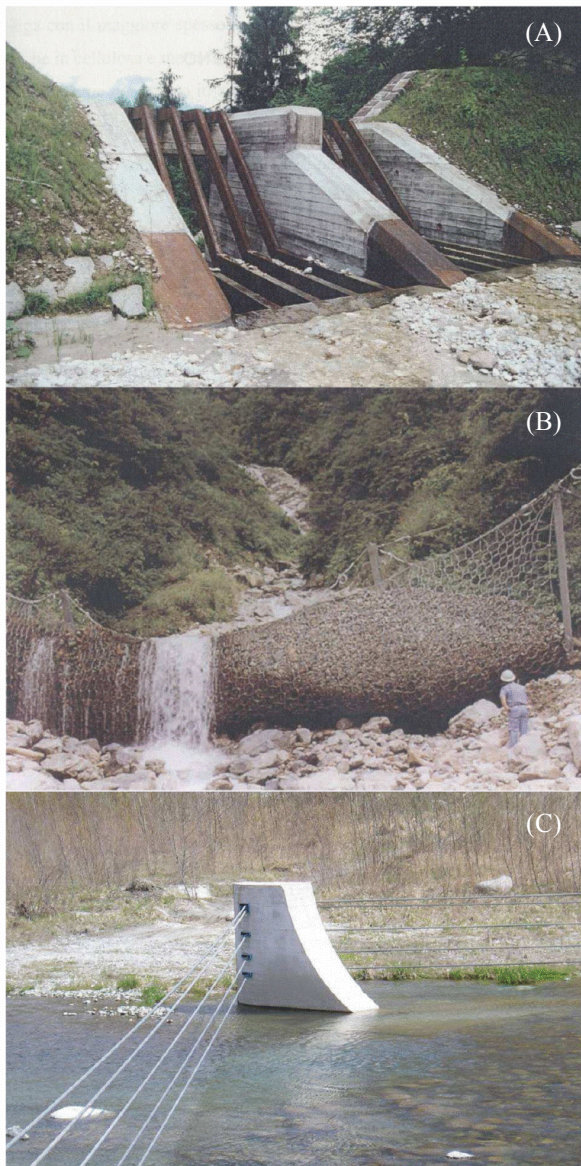
Figure 7. Wood retention control works: a filter concrete check dam (A), a rope net barrier (from: www.geobrugg.com ) (B) and a cable filter dam (C).
