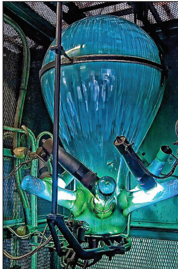
FIGURE 2 – A multinode mercury-arc rectifier still in operation in October 2010 at Manx Electric Railway substation at the Laxey Isle of Man. (Image courtesy of Tony S. at Talk Electrician Forum.)
