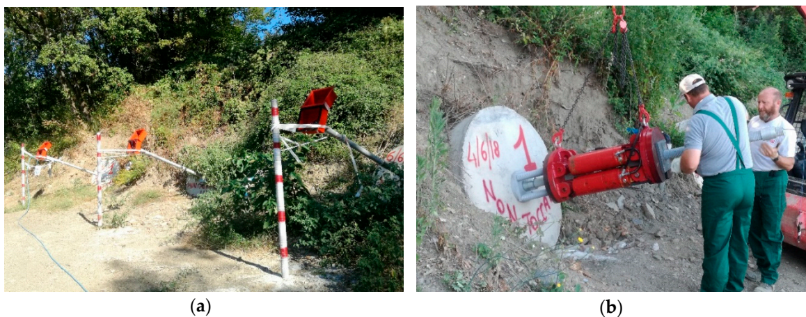
Figure 13. In-situ installation of the composite bars equipped with optical cables: (a) view of the external portion of bars with metallic boxes for hosting cables; (b) set up of the oleo-dynamic piston for the application of pre-tension to the bars.
