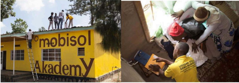
Figure 31: The Mobisol Akademie in Arusha, Tanzania, and a trained installation technician in action.
