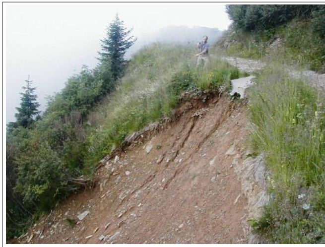
Figure 1 - Example of road induced landslide on the Eastern Italian Alps [picture courtesy of Cazorzi F.].
