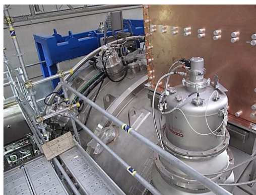
Figure 23. View of turbomolecular and cryogenic pumps installed around the SPIDER Vacuum Vessel.
