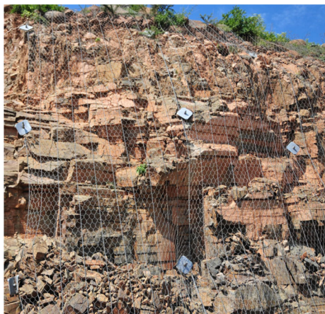
Fig. 1 Example of application of a secured drapery system (location: South Africa, courtesy of Dr. Giacchetti)
