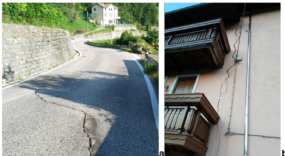
Fig. 4 Some damages caused by the Cischele landslides on: (a) the main road; (b) a house
