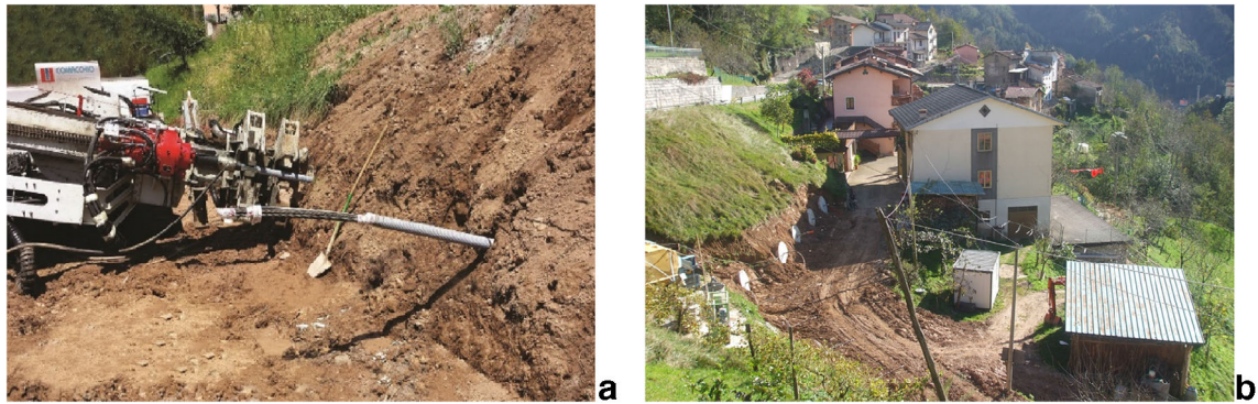
Fig. 6 Installation of composite anchors at Cischele landslide (2014): (a) Bar and strands already infixed; (b) external concrete plates of alignment B, visible at the ground surface near the house and below the road
