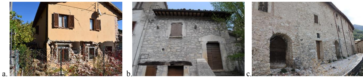
Figure 5: a) Class A building: poor masonry quality and floors replaced with rigid ones (MCC); b) C class building: random layout limestone masonry reinforced by deep repointing with cementitious mortar (CSN); c) D class building: random layout limestone masonry reinforced by grout injections and r.c. jacketing (internal side) (CMP)
