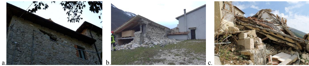
Figure 4: Examples of damage due to rigid roofs: a) Slip of the roof and horizontal arch (VZZ); b) Masonry leaves separation and local overturning (CSN); c) Total collapse due to crumbling of masonry (CMP)
