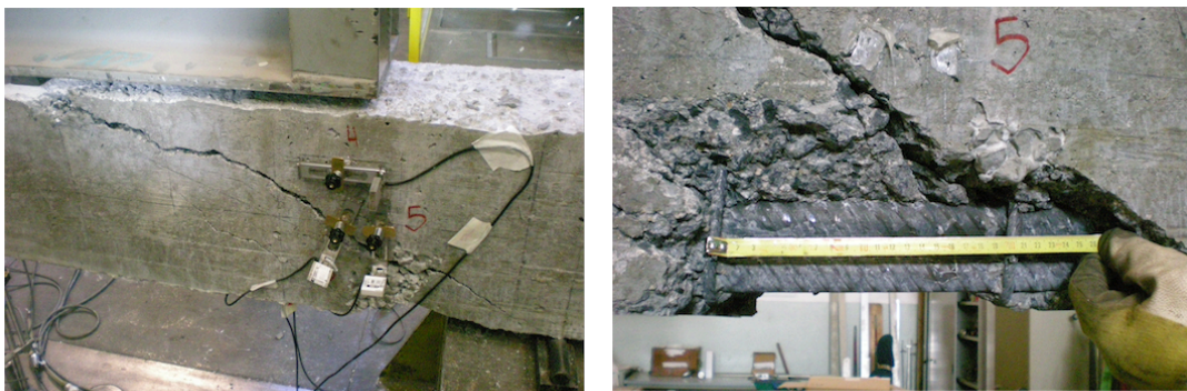
Figure 4-16. Shear failure - "B2" series.
