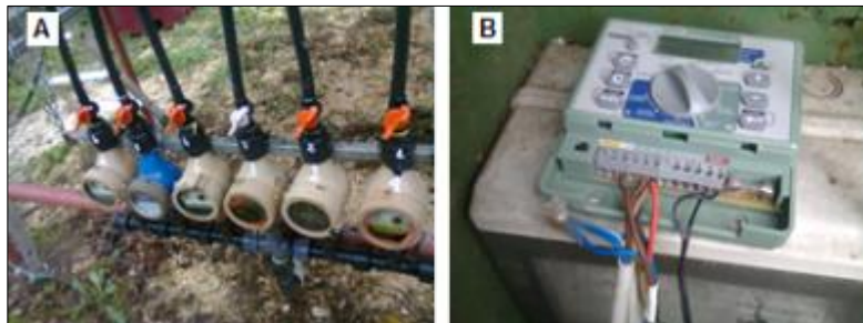
Figure 4.15 Manifold at six lines with flowmeters (A) and pump timer (B) of the CCW.
