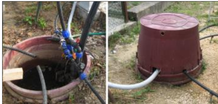
Figure 4.10 Collection tank (CT) with pumps used in 2012.
