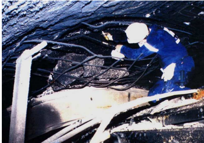
Fig. 4.1 The Great tunnel severe spalling and steel damage after the 1994 fire.
