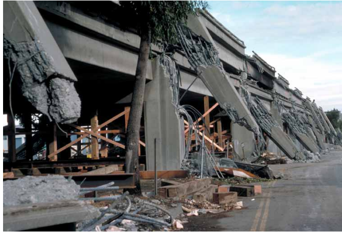
Figure 1.3: Failed support columns and collapsed upper deck of the Cypress Street Viaduct.
