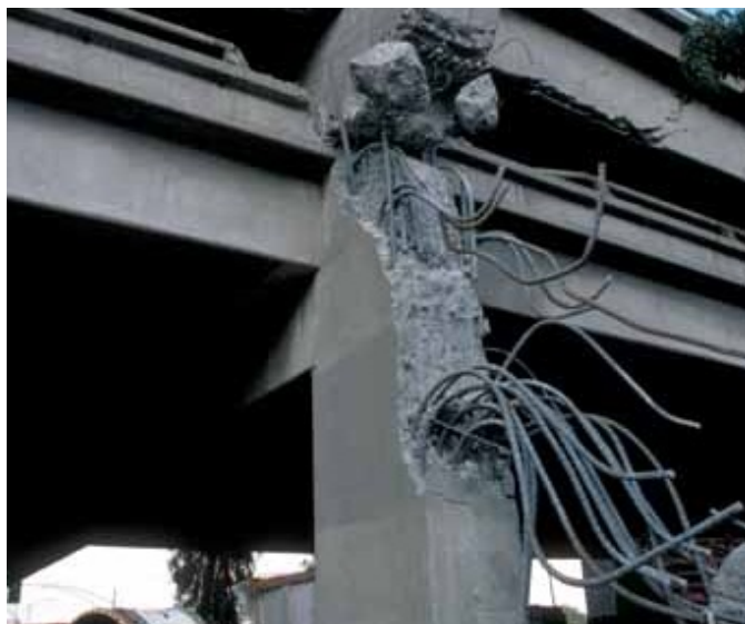
Figure 1.4: Detail of the bad anchorage of the rebar in Cypress Street Viaduct.
