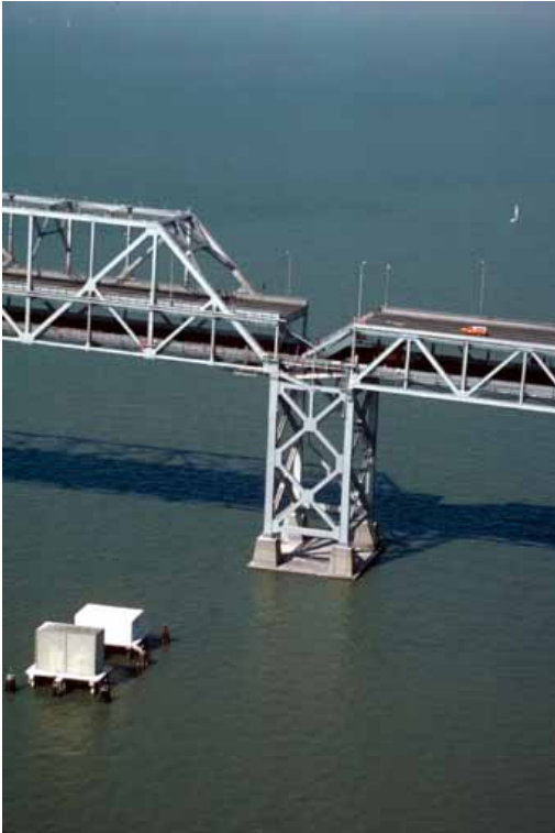
Figure 1.2: The San Francisco-Oakland Bay bridge suffered relatively minor damage. A 76-by-60-foot (23m x 15m) section of the upper deck on the eastern cantilever side crashed onto the deck below. The quake caused the Oakland side of the bridge to shift 7in (18cm) to the east. The quake caused the bolts of one section to shear off, sending the 250-short-ton (230t) section of roadbed crashing down like a trapdoor. This fault directly killed nobody, except for a driver badly instructed by road assistance personnel.
