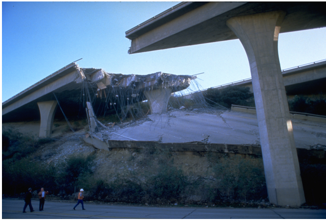
Figure 1.6: Northridge Earthquake, CA, January 17, 1994; Many roads, including bridges and elevated highways were damaged by the 6.7 magnitude earthquake. Approximately 114'000 residential and commercial structures were damaged and 72 deaths were attributed to the earthquake. Damage costs were estimated at 25 billion USD. FEMA News Photo, Author: Robert A. Eplett
