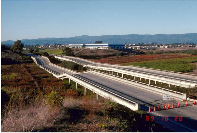
Figure 1.5: State Route 1 collapsed in western Watsonville over Struve Slough after the 1989 Loma Prieta earthquake.
