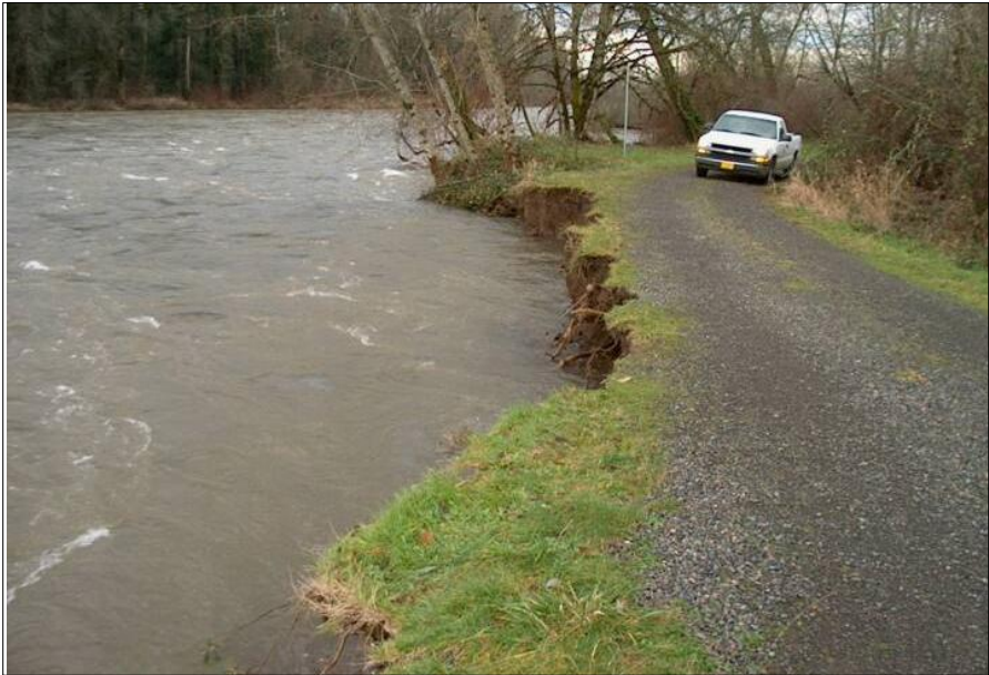
Figure 14: Impact of bank erosion on infrastructures.
