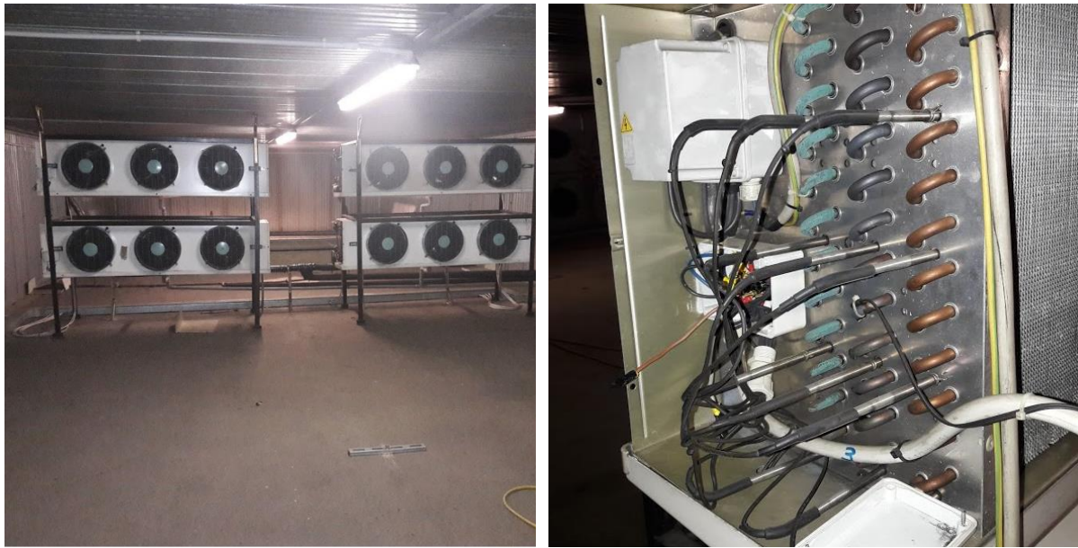
Figure 2.6 – (a) Installation of the 4 finned coil evaporators inside the machine room (b) Electric resistances for defrost operation
