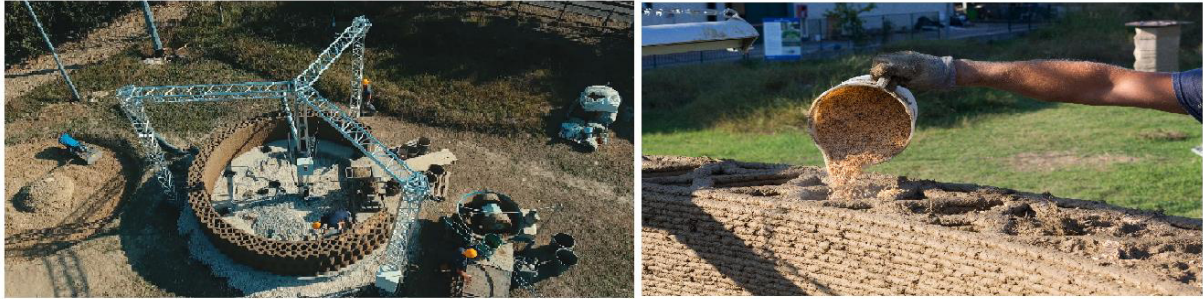
Figure 1.35. WASP Big Delta printer on the left; a detail of printed wall on the right. [58]
