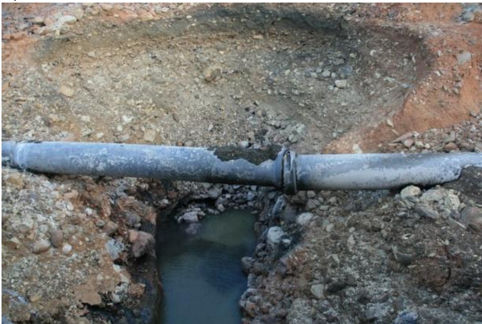
Figure 1 Crater due to natural gas pipeline explosion (La repubblica)
