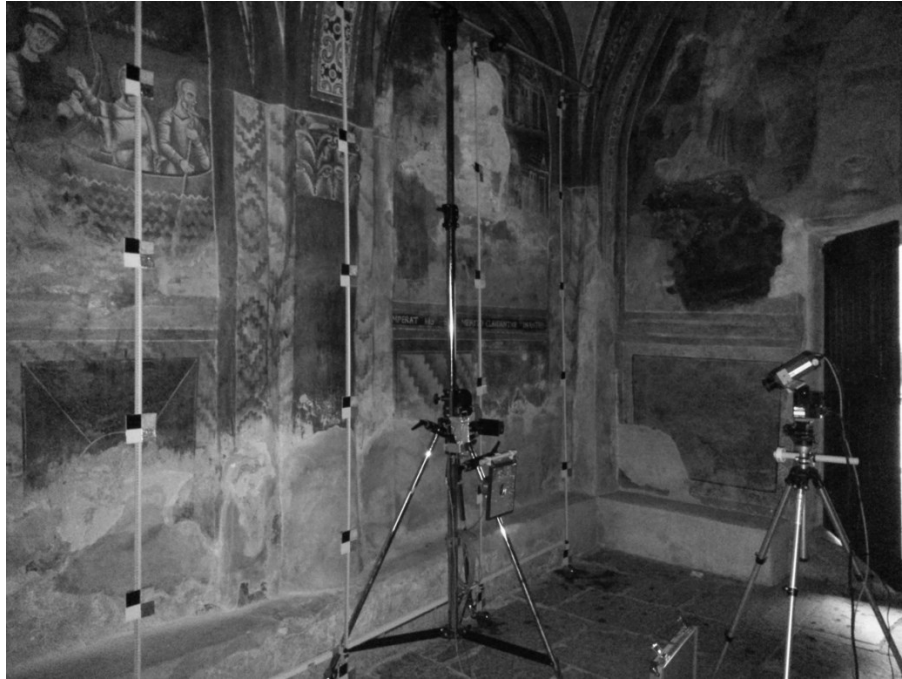
Figure 5.21: This picture shows the South wall decoration damaged in the lower part. On the right the robotized system is looking at the special reference targets placed near the wall.
