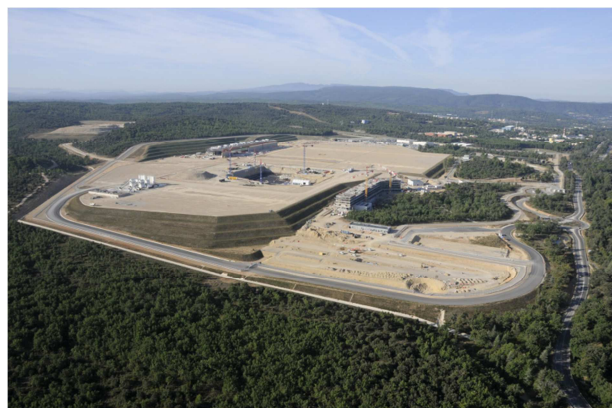
Figure 1-22: site of construction of the ITER project in Cadarache in the south of France in September 2011
