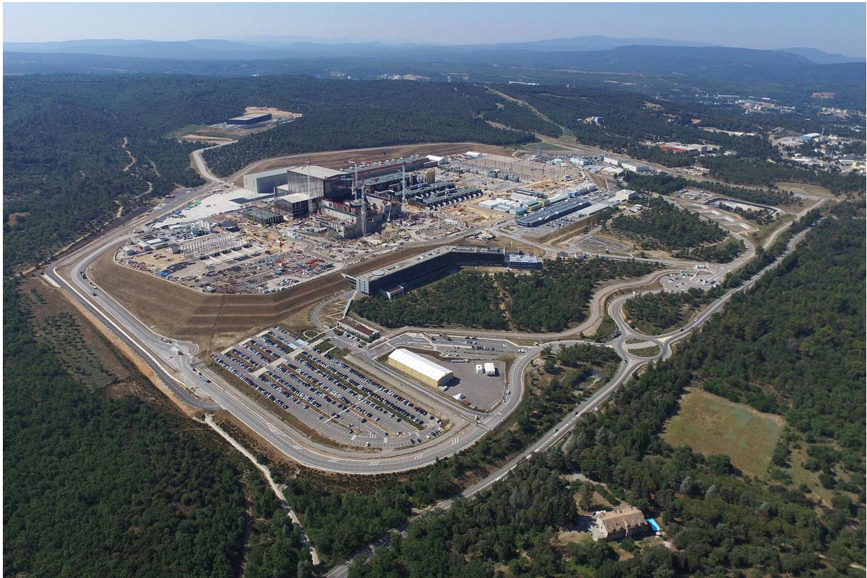
Figure 1-23: site of construction of the ITER project in Cadarache in the south of France 25 July 2018, ITER Organization/EJF Riche, https://www.iter.org/album/Media/4%20-%20Aerial
