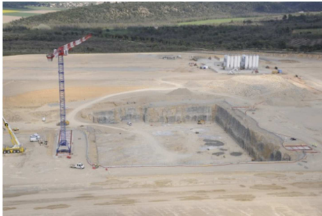
Figure 1-25: February 2011, the excavation was completed for the construction of the antiseismic platform where to build the room of the Tokamak
