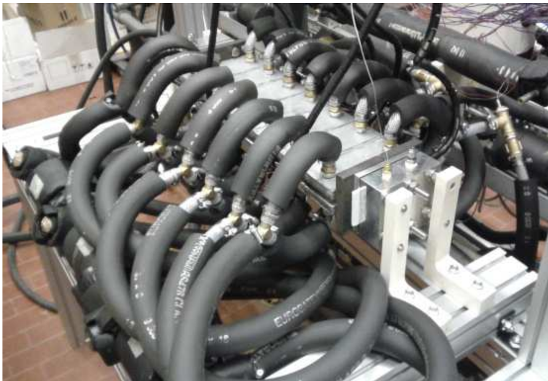
Figure 2.12. Test section with piping for the water modules.
