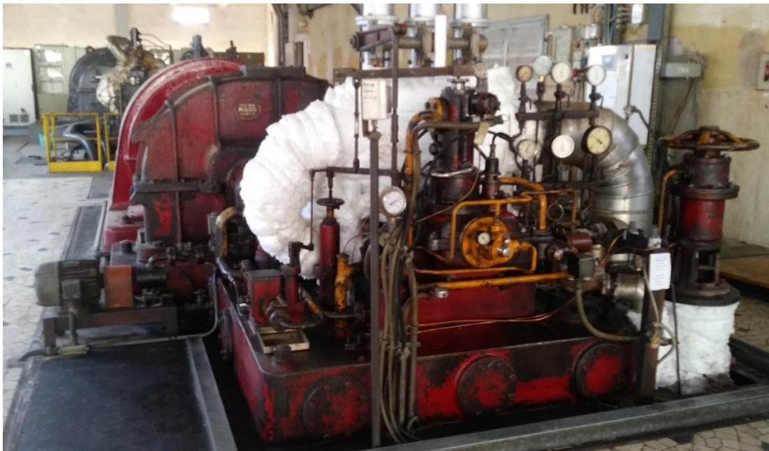
Figure 36. Photo of the existing steam turbines (turbine 1 in front, turbine 2 behind).
