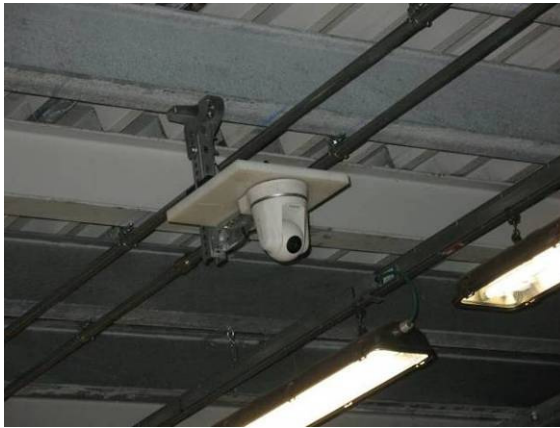
a – view of the video-camera installed on the roof of the ICE room
