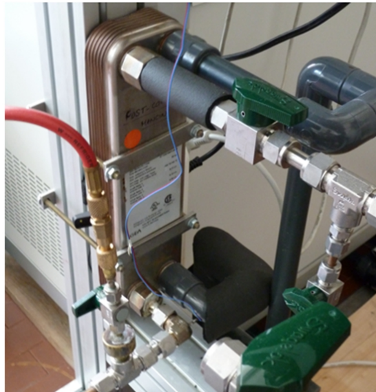
Figure 4.28: Picture of the sink water loop.
