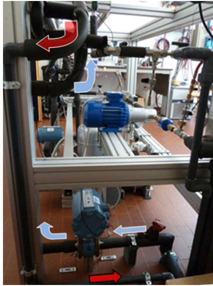
Figure 4.27: Picture of the cold water loop.
