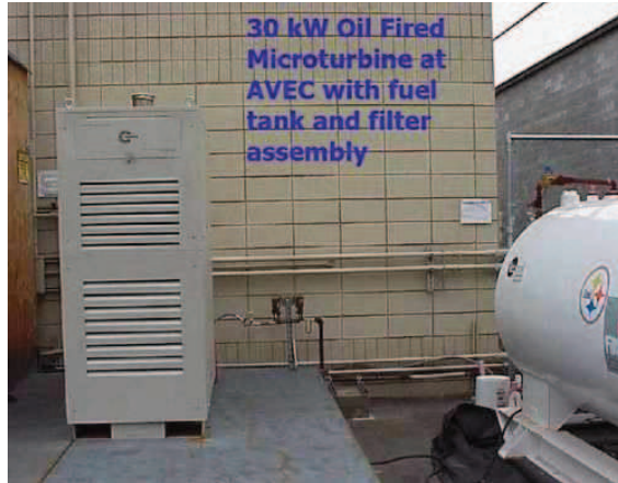
Figure 2.5: 30 kW Oil Fired MT with Fuel tank and Filter assembly.
