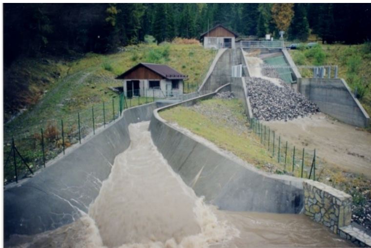
Figure 22: Monitoring station of Rio Cordon.
