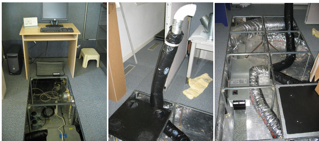
[Figure 2.3, 2.4, 2.5: Raised floor in the CEC and flexible ducts that connect the system to the desk-mounted PVS.]
