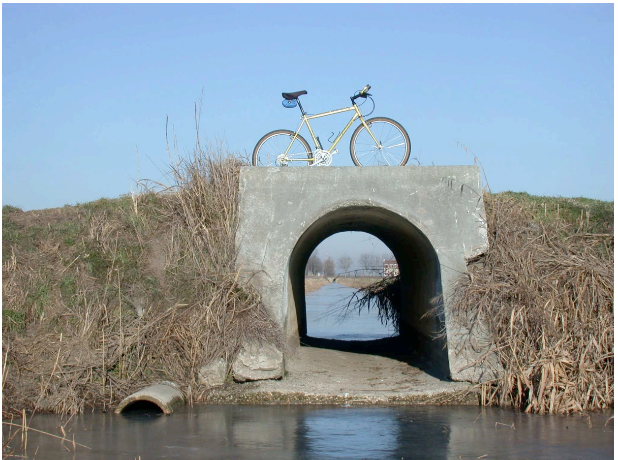
Figure 2.4: Bridge with culvert, whose foundations currently above the channel level prevent the water flow.
