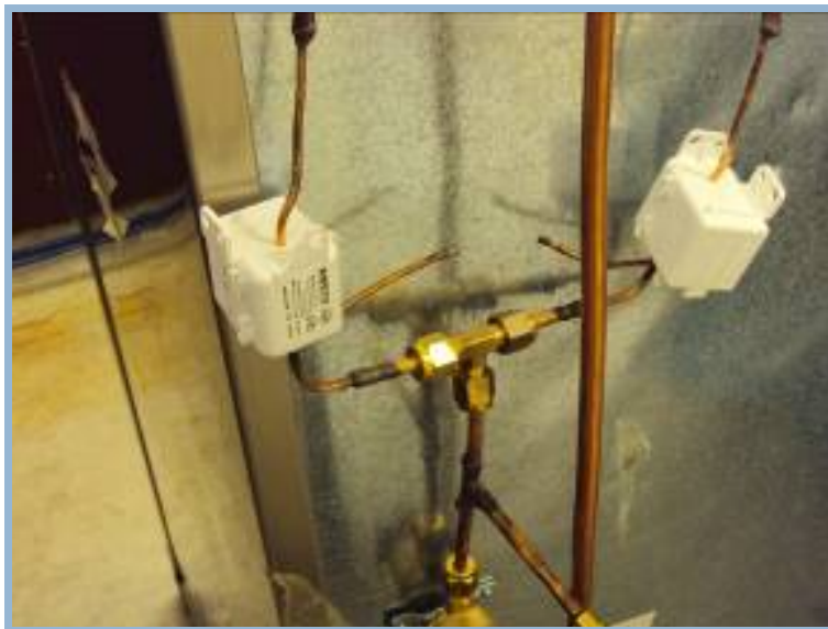
Figure 3.3.9 Solenoid valves after the dryer
